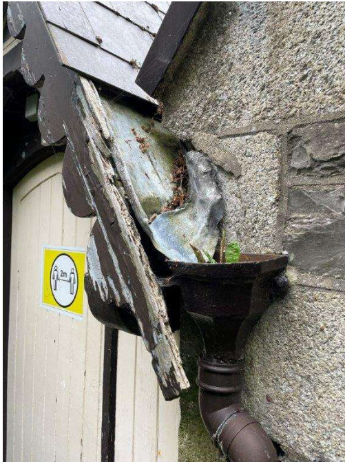
Fig. 06: Water ingress resulting in deterioration of decorative fascia to door at eastern elevation.
