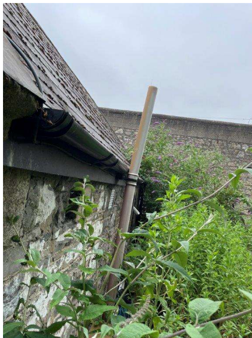
Fig. 07: Moss visible on roof slates at northern elevation.
