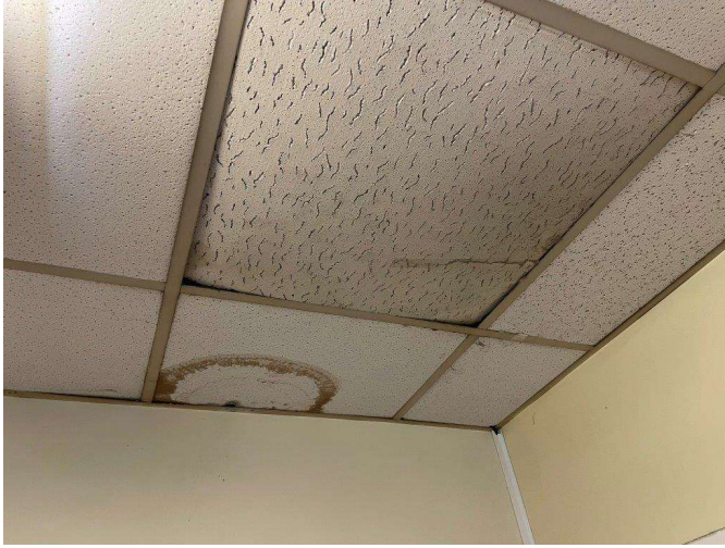
Fig. 10: Deterioration/rot of suspended ceiling panels inside Gate Lodge due to water ingress.
